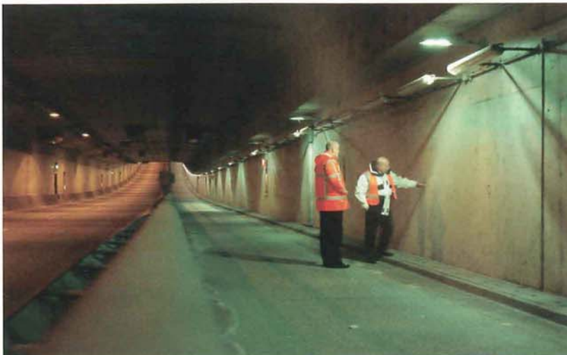
3600 Watt replaced by 160W in total
